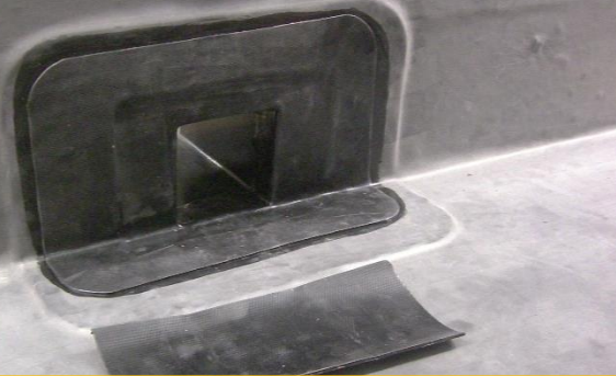
Cut additional piece of Elasto-form to fit inside of outlet and apply primer to bonding area
